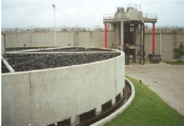
Photo: Tricking filter and UASB
